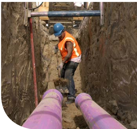
Recycled water, distributed through purple pipe, is one of the ways CUWA agencies are diversifying their supply portfolios.
